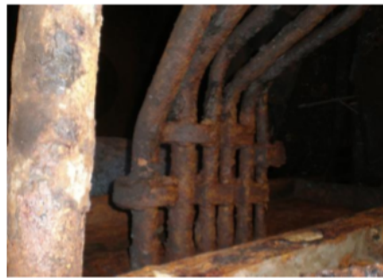
FIGURE 1. Corrosion on gas pipeline
