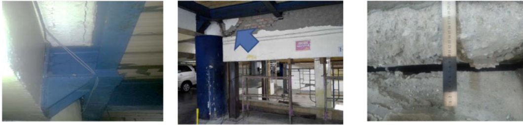
Figure. 2. Damage to the upper structure
