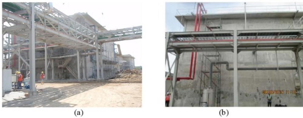
Fig. 1. Waste water treatment building: (a) condition of the plant and (b) the 12 m reinforced concrete wall.
