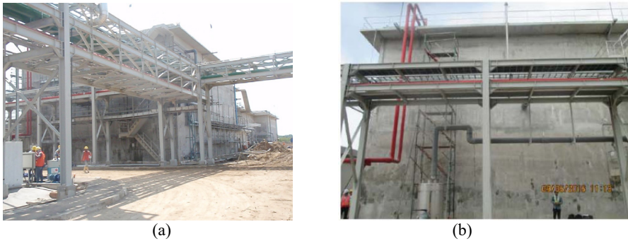
Fig. 1. Waste water treatment building: (a) condition of the plant and (b) the 12 m reinforced concrete wall.
