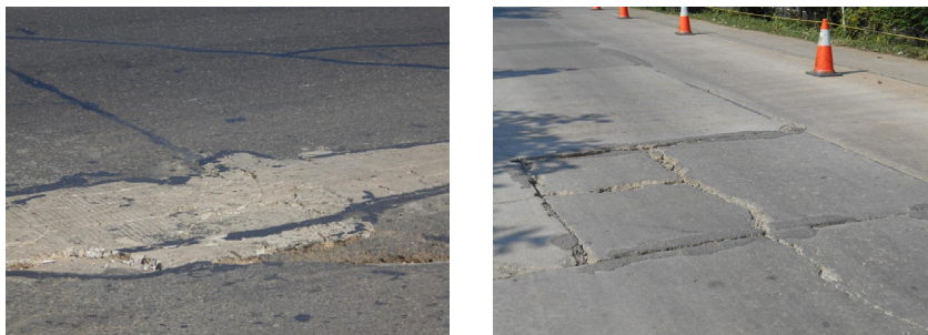
Fig. 1. Damage to the rigid pavement.
