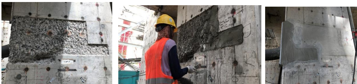
Figure 2. Honeycomb from 10 mm up to 10 mm upto less than 50 mm and concrete cover less than 40 mm
