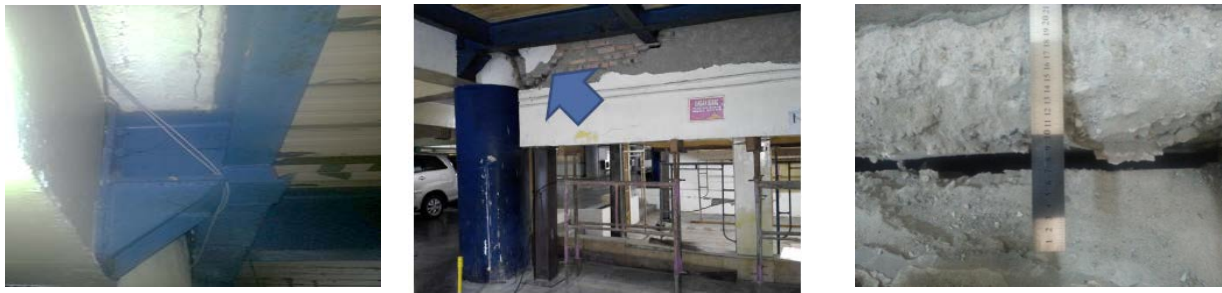
Figure. 2. Damage to the upper structure
