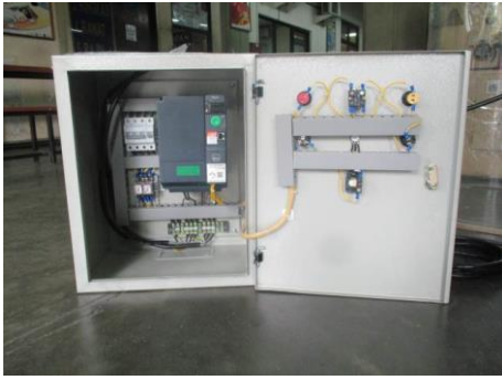
(a) Panel Listrik
