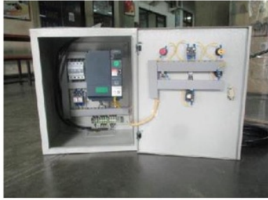
(a) Panel Listrik
