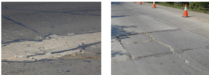
Fig. 1. Damage to the rigid pavement.
